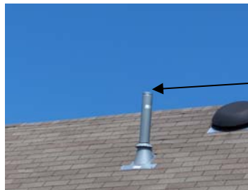
Flue cap missing (Replace)
